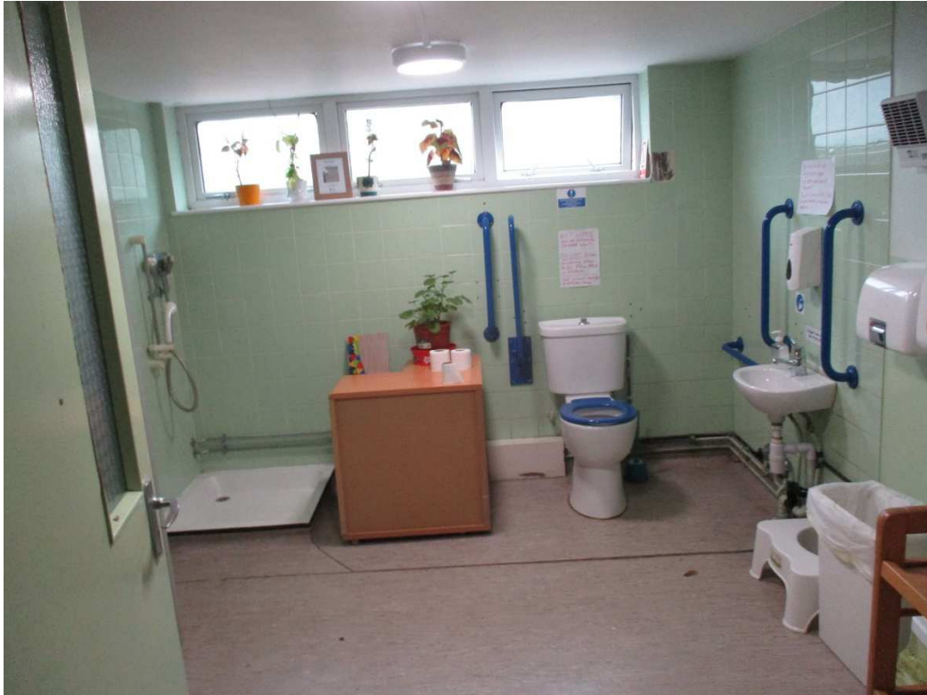
Photo 18 – Existing WC/ shower facility/ Proposed upgrade to Changing Places WC Low ceiling height will prevent install/ use of tracked hoist.
