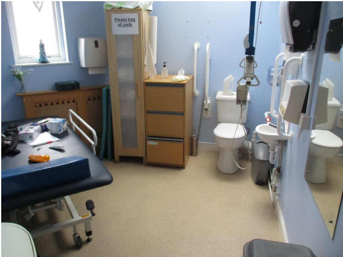
Photo 5 – WC with hoist and changing bed. Restricted manoeuvring space/ room undersized. WC in corner does not allow for assistance from either side
