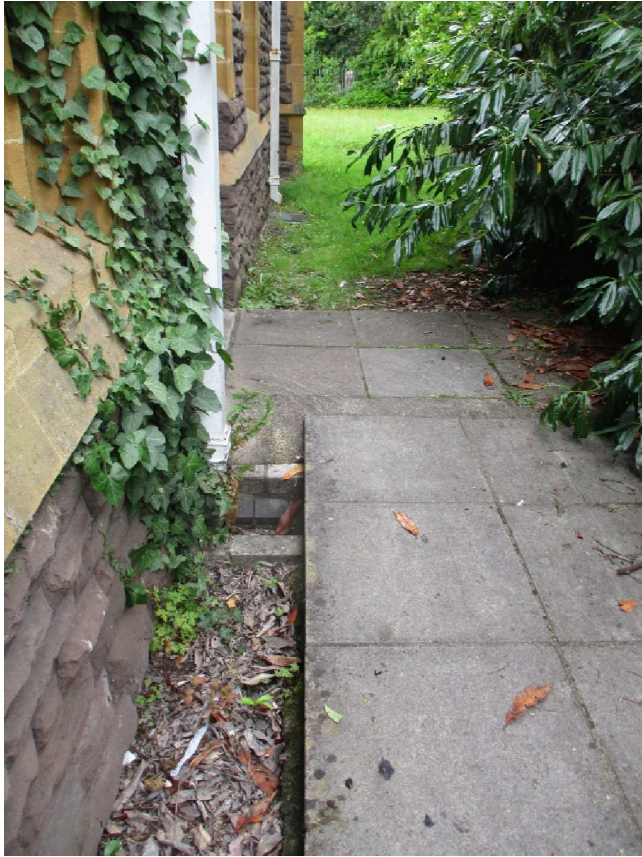
Photo 9 – Drop off at edge of path.
