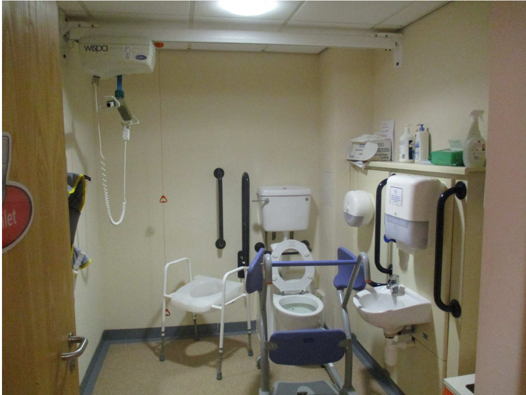
Photo 26 Corner layout Accessible WC, with various toileting aids and tracked hoist.
