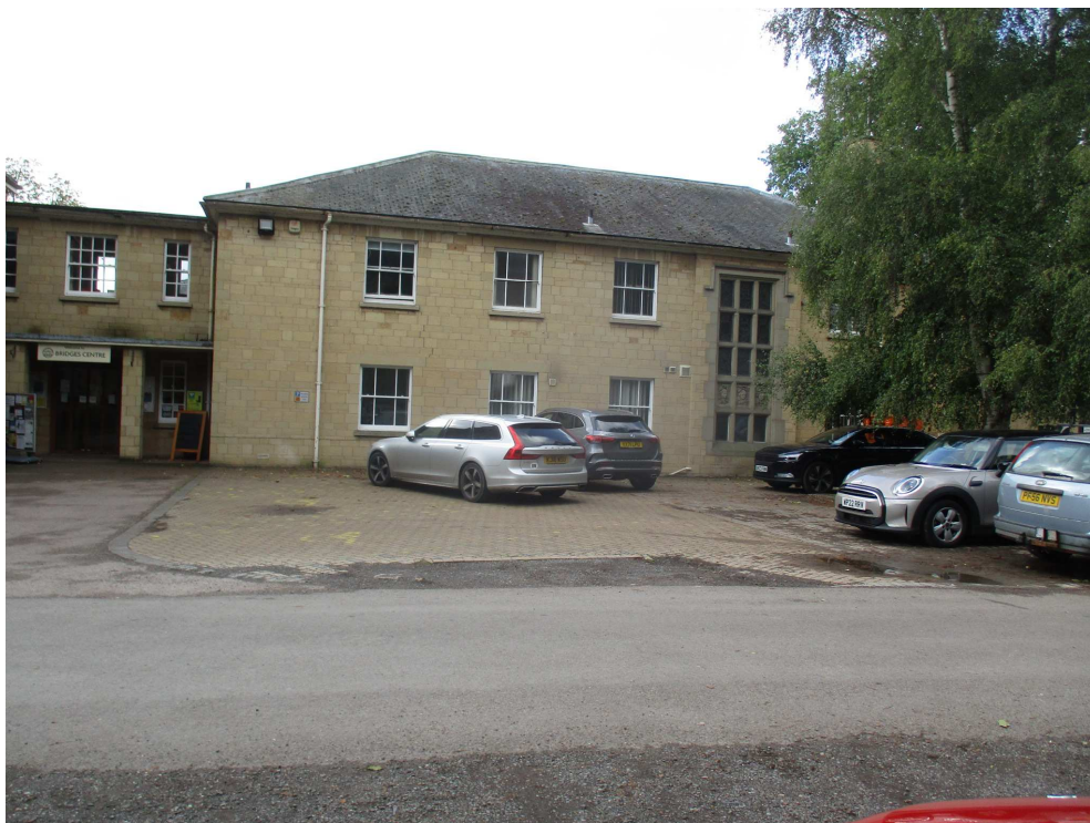
Photo 29 Some uneven surfacing to parking area.
